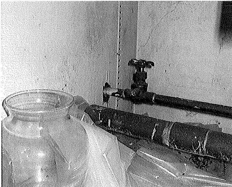
Space around sink pipe
