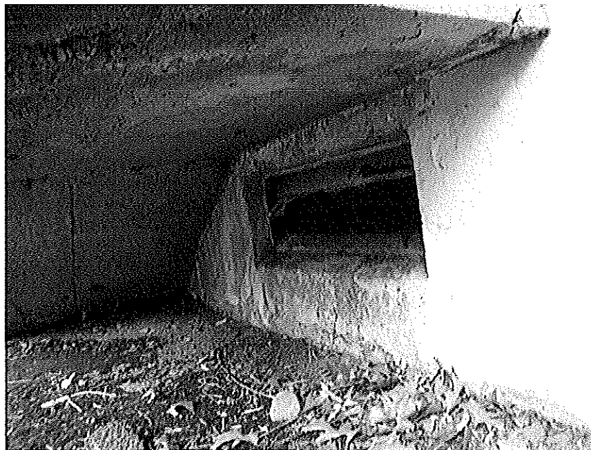
Crawlspace exhaust vent below staircase
