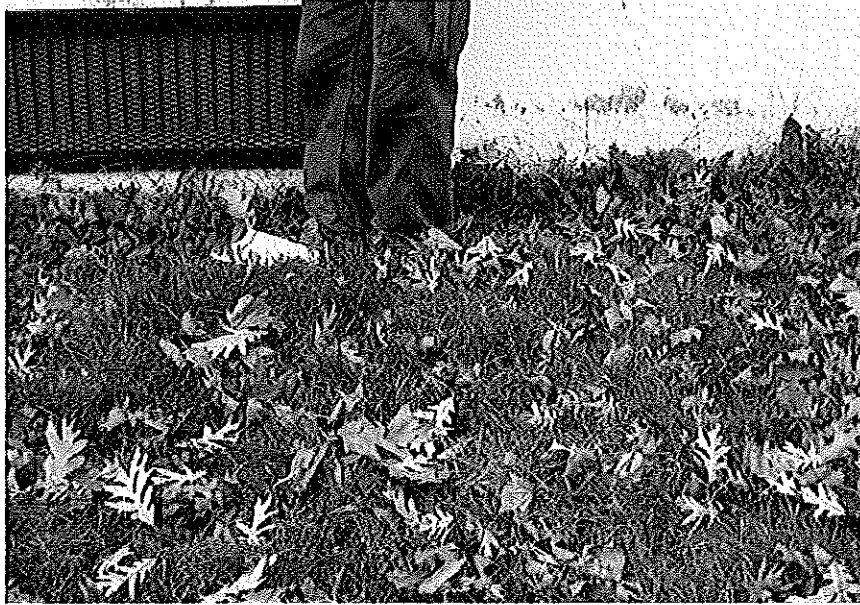
Depression in soil near footing to building (note level of grass in foreground and lack of visibility of feet in background)
