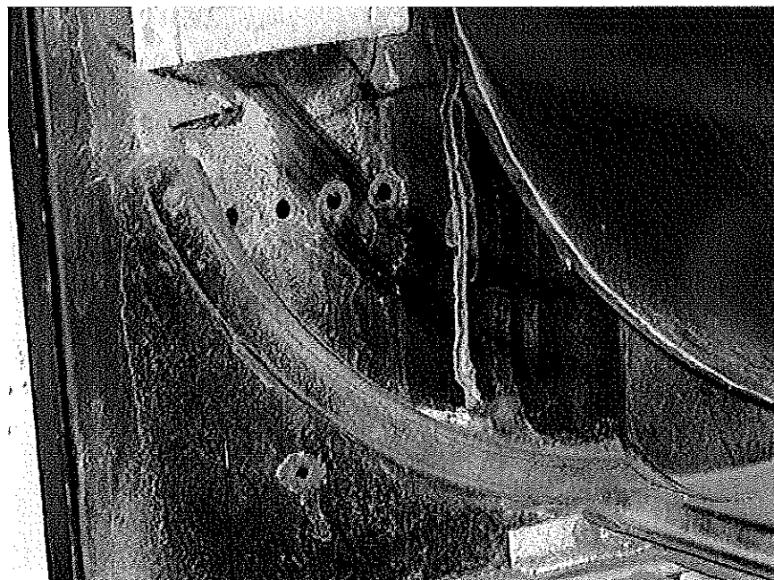
Holes in univent cabinet wall
