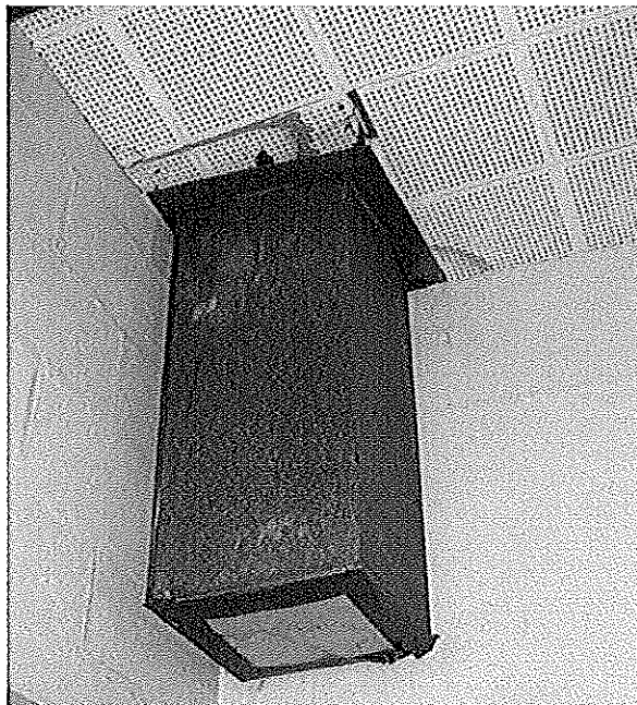
Cardstock-sealed vent, note water-damaged interlocking ceiling tiles
