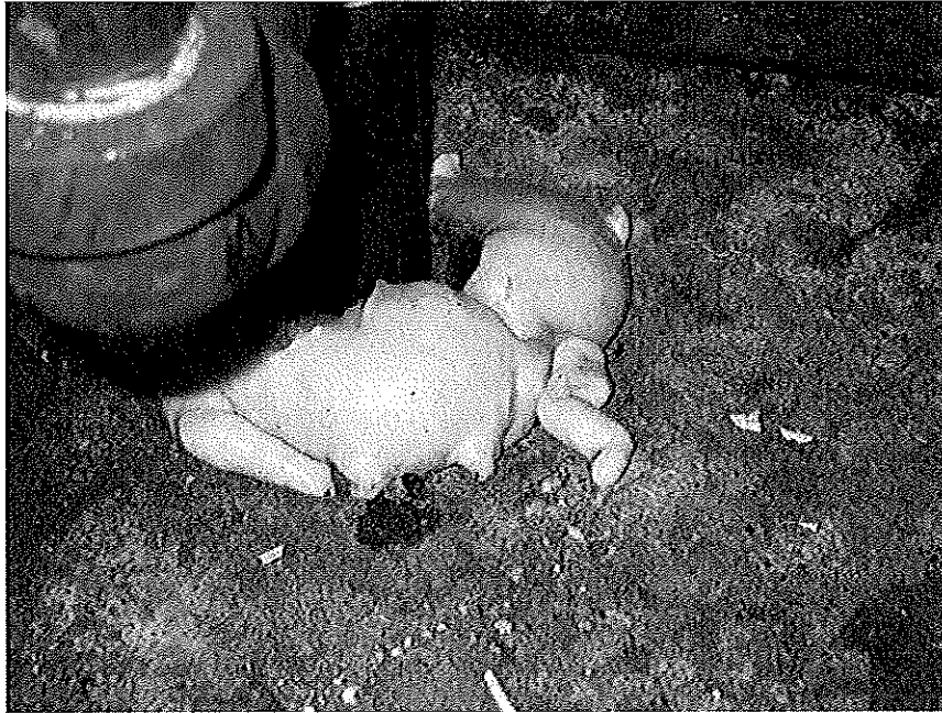
Space around pipe (with deteriorating old spray foam)
